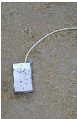
Not just a trip hazard ... the casing is damaged too!
